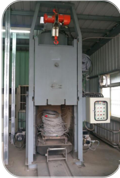
RESOURCE RECOVERY FURNACE
