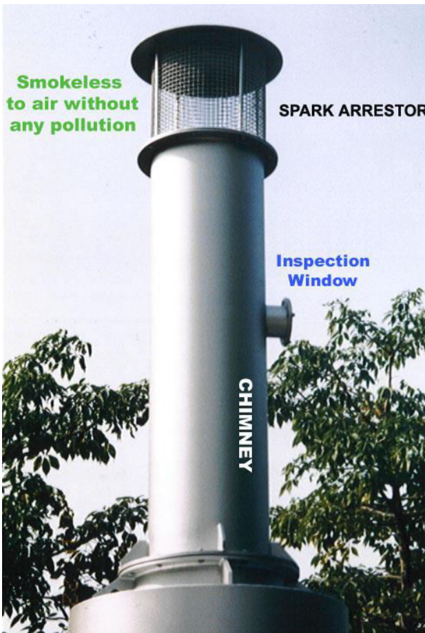
SS #304 CHIMNEY WITH HEAT RESISTANT PAINTING
