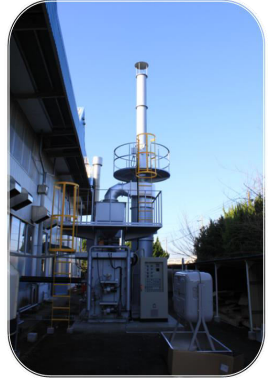
WASTE LIQUID FURNACE
